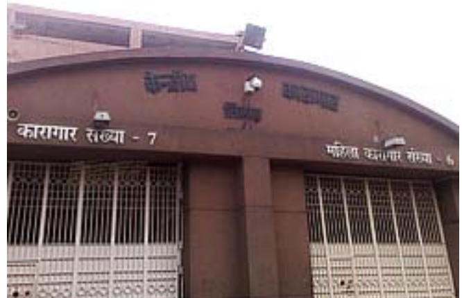
Bosch AutoDome camera installed at one of the Prisons of Tihar Jail.
